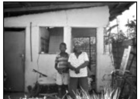
Octavius' former home, damaged by the earthquake, is now used for storage
