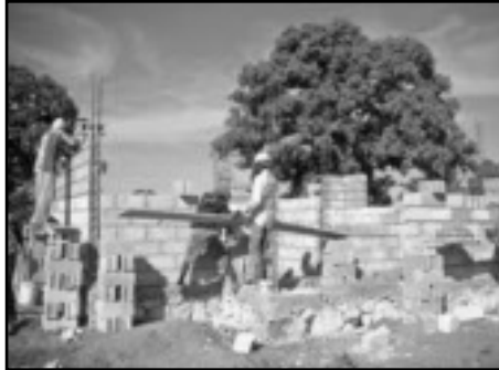
Construction workers use string to measure even layers of block, ensuring homes are straight and strong
