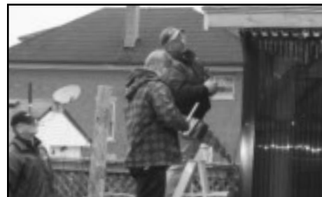
Simcoe Lions Dave Stelpstra (left), Scott Dawson and Ron Francis work on an enclosure for a therapy spa for a Norfolk teenager. Clubs from Vittoria, Port Dover and Simcoe teamed up with money and know-how to help Alex Kirton, who was born with Peters' Anomaly and experienced development delays because of his blindness, enjoy physical activity from the hot tub
