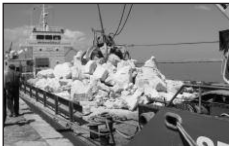
Lions have tackled huge environmental projects for decades. A Lion in Italy played a key role in submerging barriers to prevent erosion
