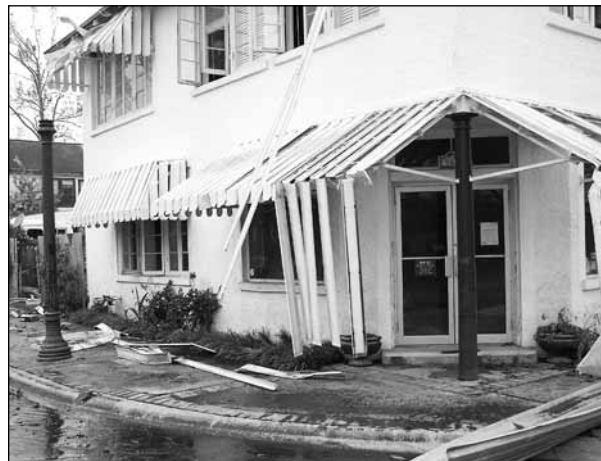
DuBuisson's dry cleaning business was irreparably damaged by the storm.
