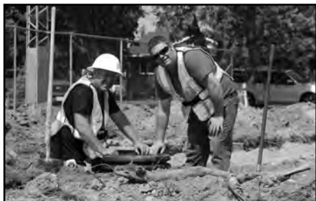
Atwood Lions members Tim Buchanan and Lion President Jeff Erwin work to ensure proper drainage is in place for the outdoor rink
