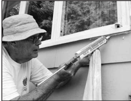
Charles Mills of the Austin Noon Lions Club in Minnesota caulks a window at the home of Norene Sundal
