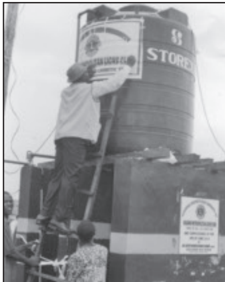
Sagamu Metropolitan Lions sank a borehole equipped with an overhead tank and power generator to supply water to residents of Ogijo in Nigeria
